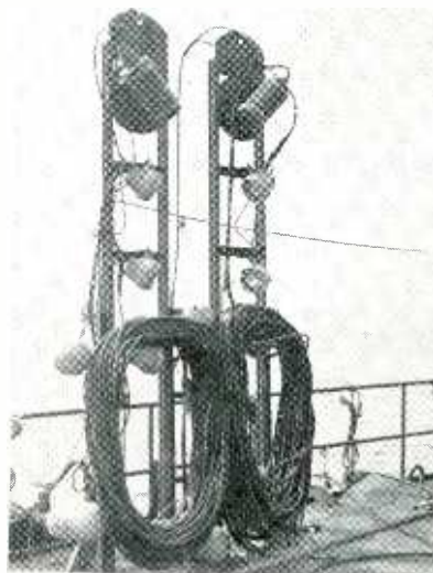
Saddle rig mounting two tv cameras and eight 500-w spotlights. This device travels along the pipe as it is being connected under water
